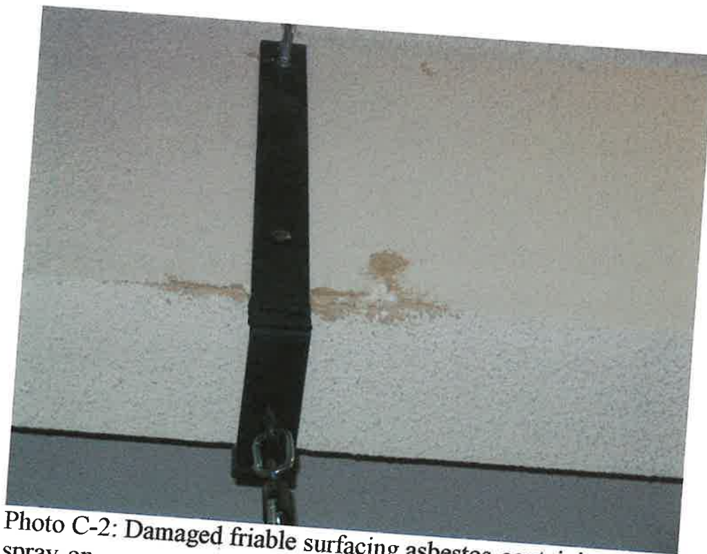
Photo C-1: Damaged friable surfacing asbestos-containing ceiling acoustic spray-on.
